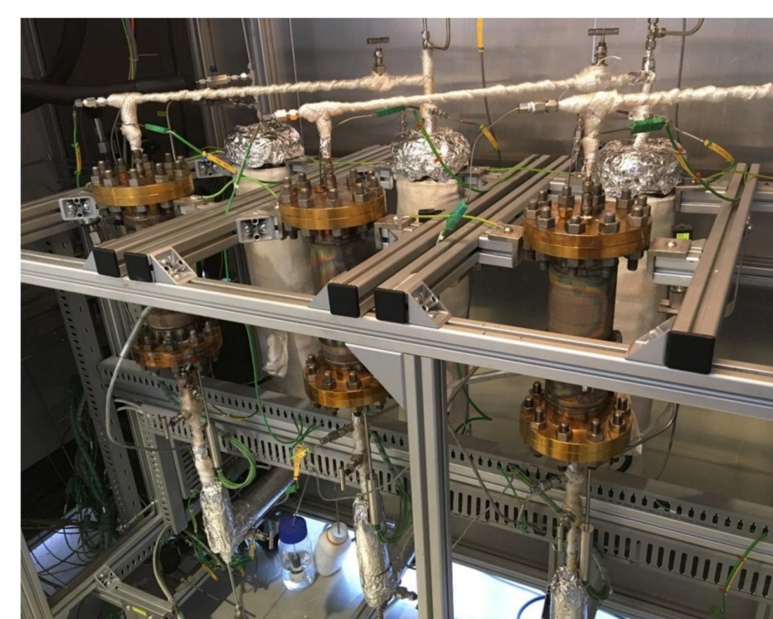
Fig. 2: Methanation test rig at MUL
